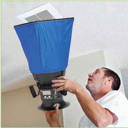
Balometer used to verify installed performance
