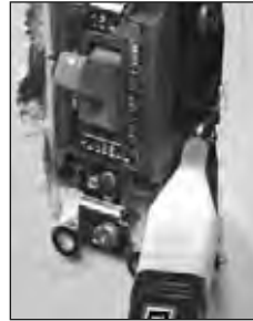
AC Voltage in switches
