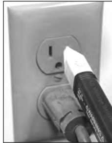
AC Voltage in wall receptacles
