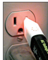
AC Voltage in wall receptacles
