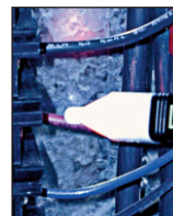
AC Voltage in junction boxes
