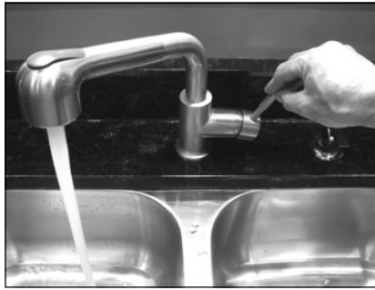
Figure 46: Let the hot water run until it is cool.
