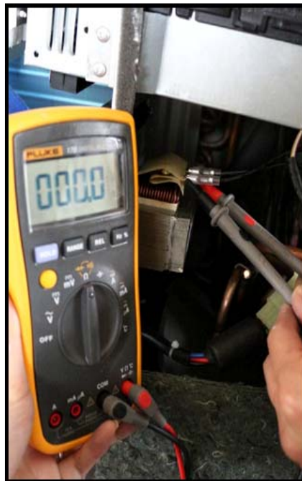
Fig. 33 – Test the Reactor Resistance
